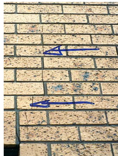
Figure 29j – Reference House R8 (Jewell) – vertical crack brick
