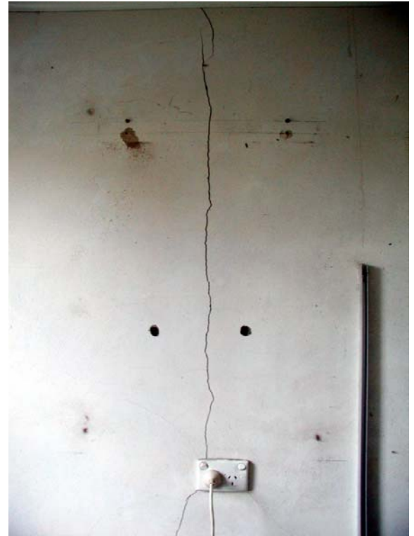
Figure 21f – Close up of vertical crack in rendered finish in laundry (Figure 21e)
