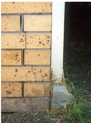
Figure 29e – Reference House R7 (Cessnock) – diagonal brick crack
