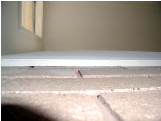
Figure 21a- Bulging plaster above the stairs
