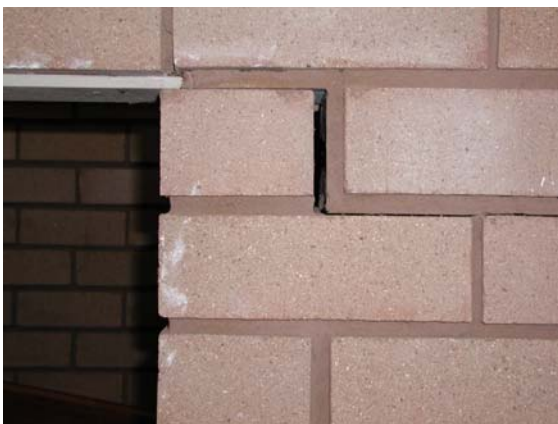
Figure 21c – Close up of Tapered stepped crack in brickwork at entrance (Figure 21b)
