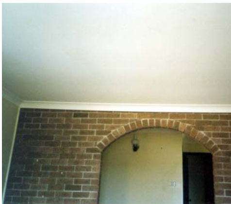
Figure 15a - Sagging lounge room ceiling after a PPV of 70 mm/s
