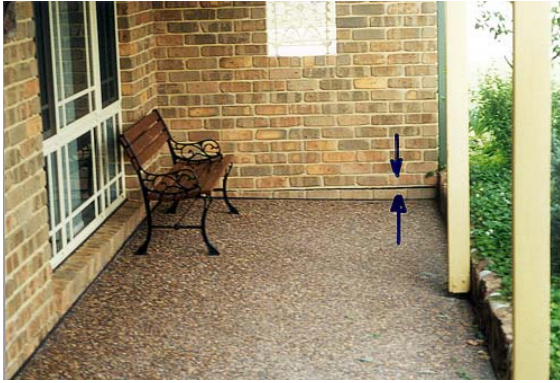
Figure 29a – Reference House R2 (Edgeworth) – bed joint separation
