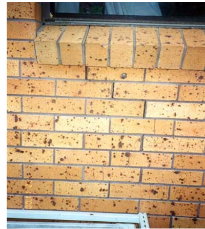
Figure 29d – Reference House R7 (Cessnock) – diagonal brick crack
