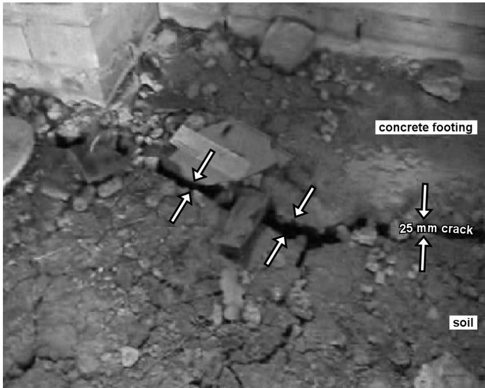
Figure 6 - 25 mm crack between footing and soil beneath house
