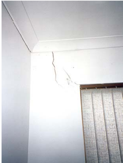
Figure 29m – Reference House R8 (Jewell) – lining and cornice crack
