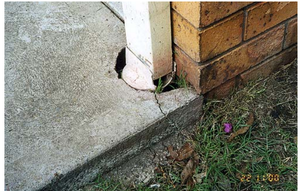
Figure 29p – Reference House R7 (Cessnock) – relative movement and slab crack
