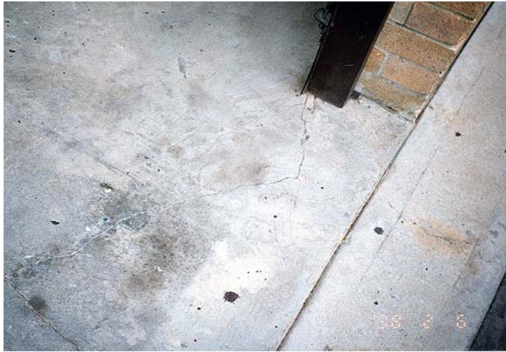
Figure 29s – Reference House R4 (Fennell Bay 2) – slab crack
