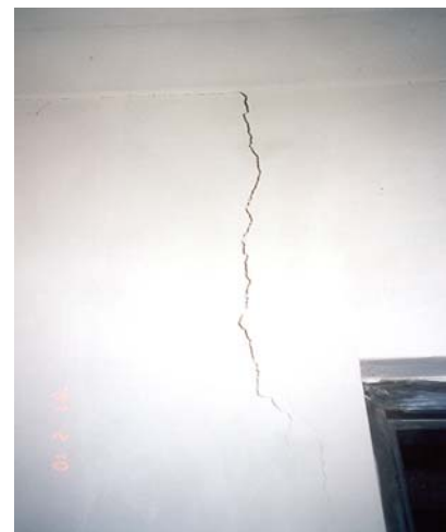
Figure 29l – Reference House R8 (Jewell) – rendered masonry crack
