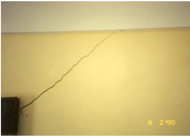
Figure 3q - 45° plaster crack in laundry
