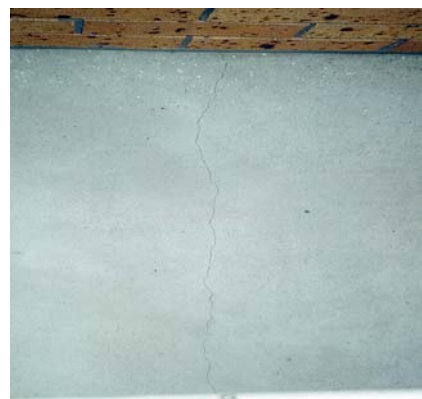
Figure 29r – Reference House R8 (Jewell) – slab crack
