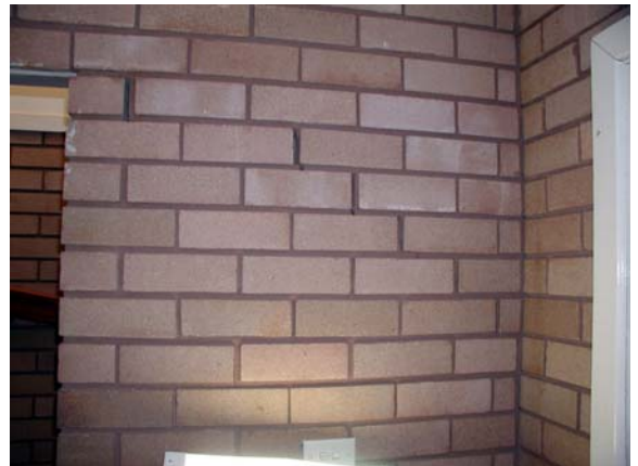
Figure 21b – Tapered stepped crack in brickwork at entrance (up to 8 mm wide)
