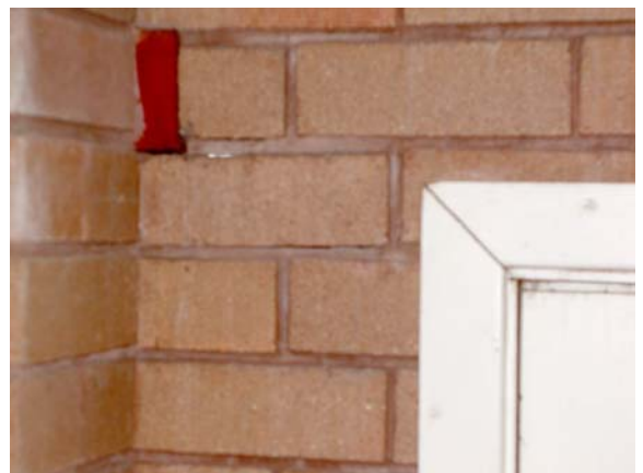
Figure 21d – Cracks in brickwork over door in rumpus room
