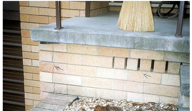
Figure 29h – Reference House R4 (Fennell Bay 2) – foundation brick crack
