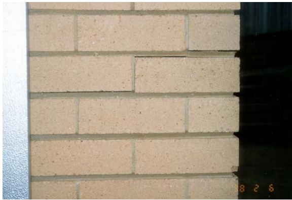
Figure 29c – Reference House R4 (Fennell Bay 2) – brick crack
