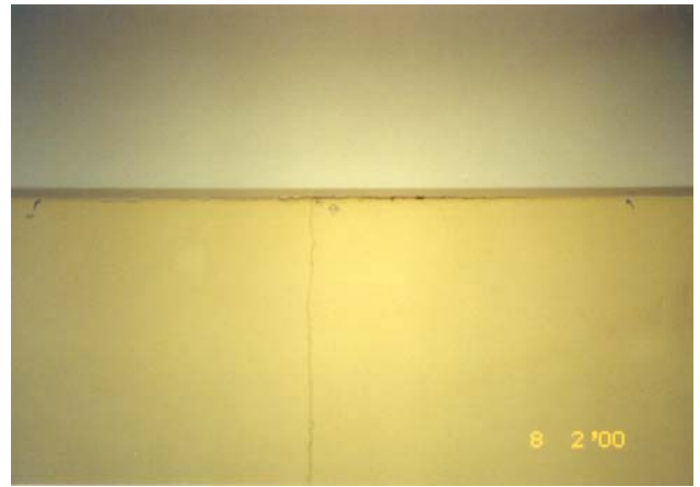
Figure 3r - Cracked cornice/wall and plaster sheet join, laundry
