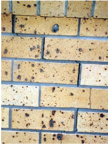
Figure 29g – Reference House R8 (Jewell) – diagonal brick crack
