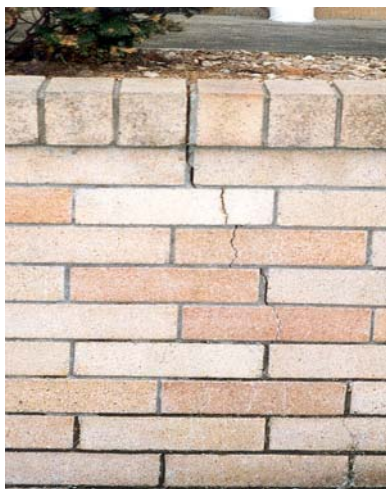
Figure 29k – Reference House R4 (Fennell Bay 2) – vertical crack brick
