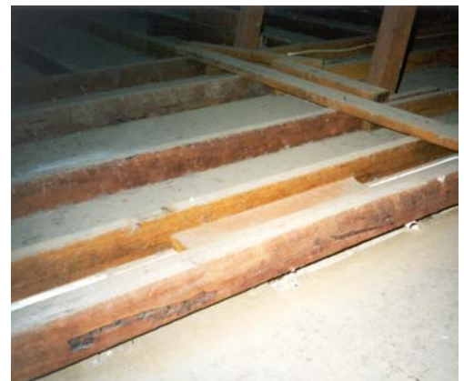
Figure 15b – Lounge room ceiling - nails pulled through plaster and backing paper causing the ceiling to sag
